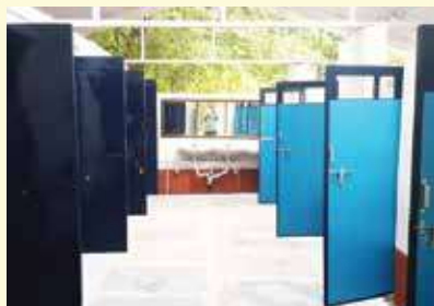
Construction of Toilets The Timbaktu Collective for the Nature School Andhra Pradesh
